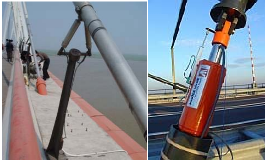
Figure 2-9 MR damper installed on cable-stayed bridges
