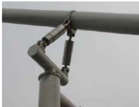
Figure 2-12 Two oil dampers installed on second Nanjing Yangtze Bridge
