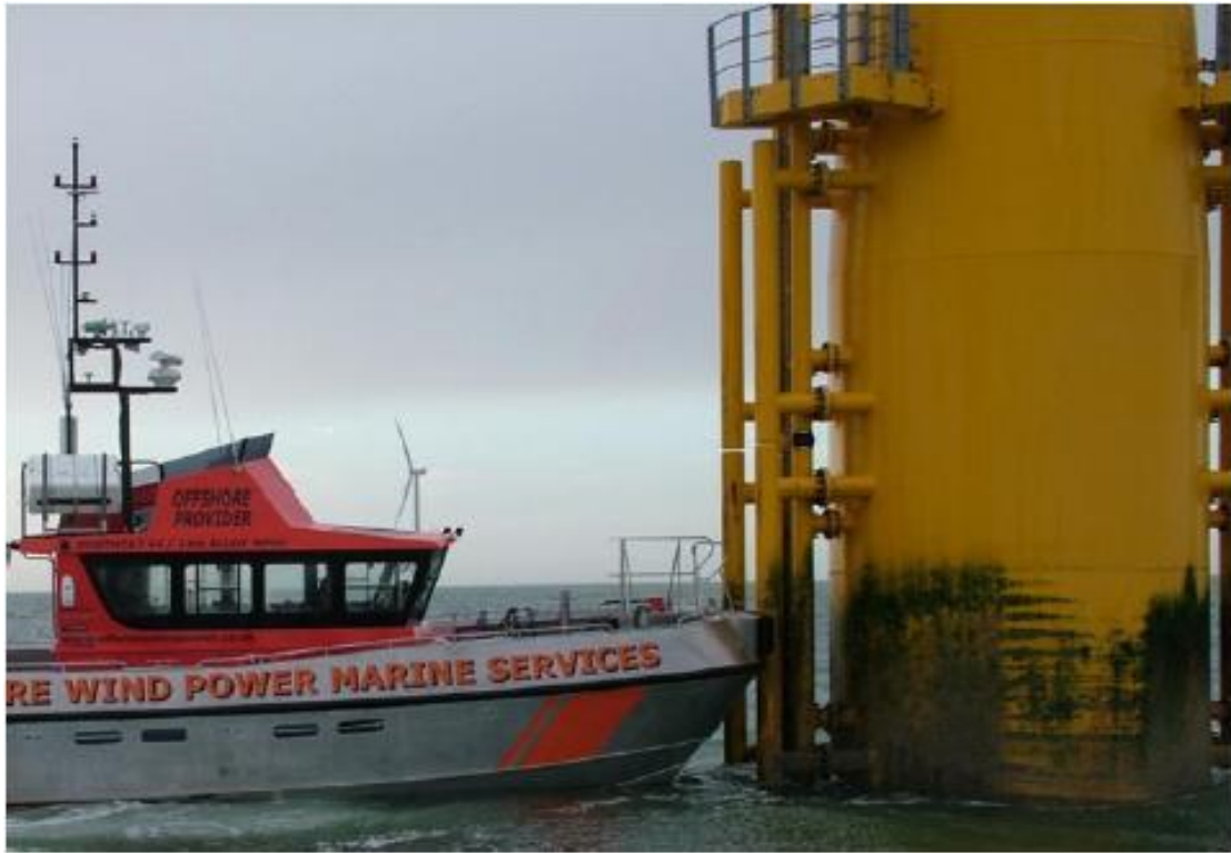
Figure 7 Servicing of offshore wind turbine with corroded base. Image courtesy of Ciang et al. [80].
