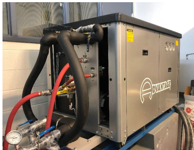
Figure B. 3. Chiller
