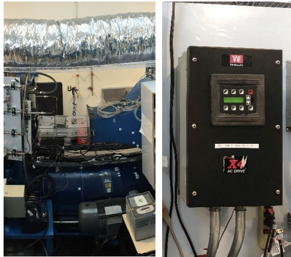
Figure B.4. Air blower and controller
