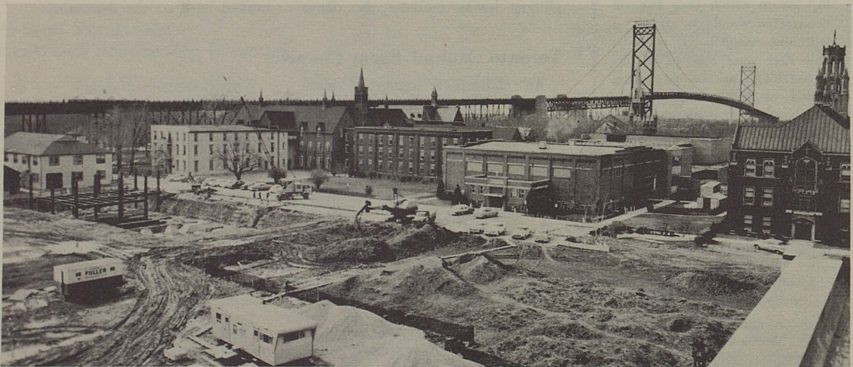
This view of the campus taken from the top of the Essex College building, shows the location of Cody Hall (steel framework in lower left) and the University Centre (behind St. Denis Hall in the corridor formed between that building and Dillon Hall). When Cody Hall is completed, the area traditionally known as "The Little Walk" will be made into a landscaped quadrangle.
