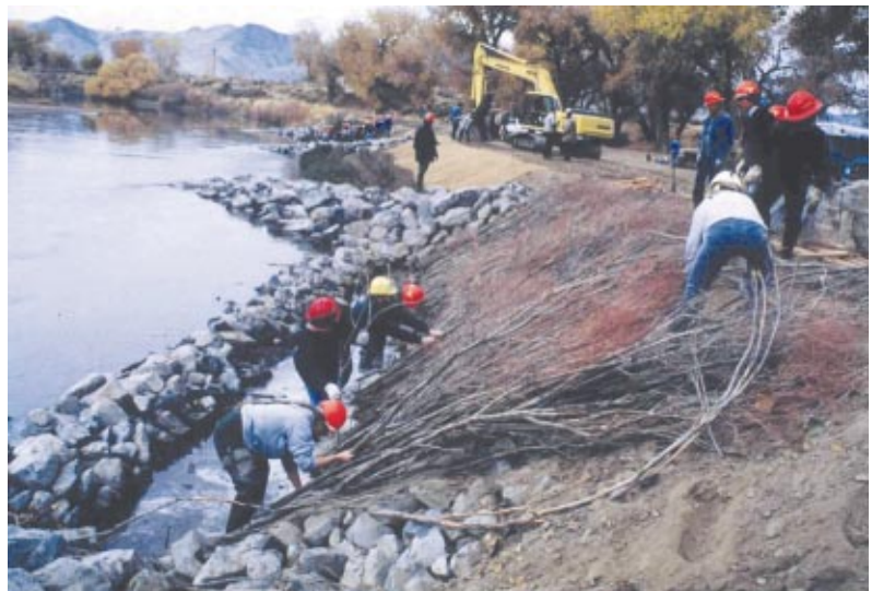
Figure 34 The willow brush trench between barb three and refusal. No erosion control blanket is used.
