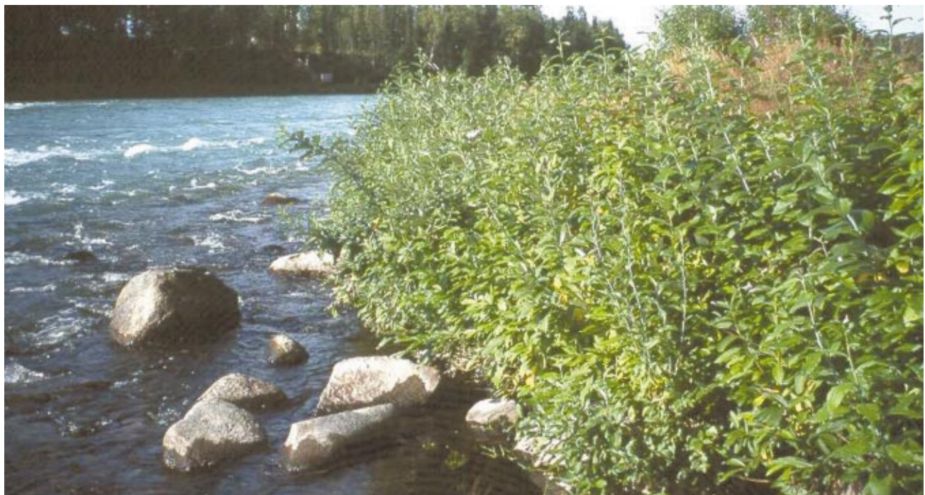
Figure 15 Large rocks placed in front of the live cribwalls provided additional fish cover.
