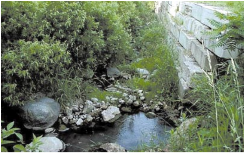
Figure 40 Deterioration of the concrete block wall, showing undermining and slumping of the structure on June 28, 2000.
