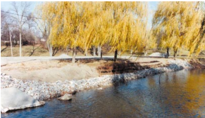
Figure 37 The workshop construction area where the three various techniques were used (from left to right: the brushmattress, vegetative geogrid, and live fascine).
