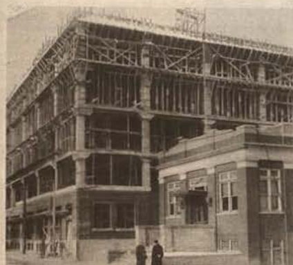
THE OLD GIVES WAY TO THE NEW. Photograph shows the six-storey building under construction (completed in 1914) To make way for it, the former Walkerville Wagon Works was torn down.
