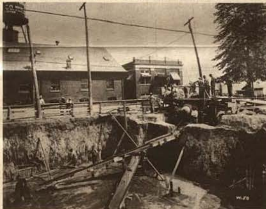
EXCAVATING FOR BUILDING 1J. The picture was taken in 1912, although the building was not finished until 1914. Note the original Walkerville Wagon Works, which was torn down in 1914, but prior to that, used as a receiving depot.
