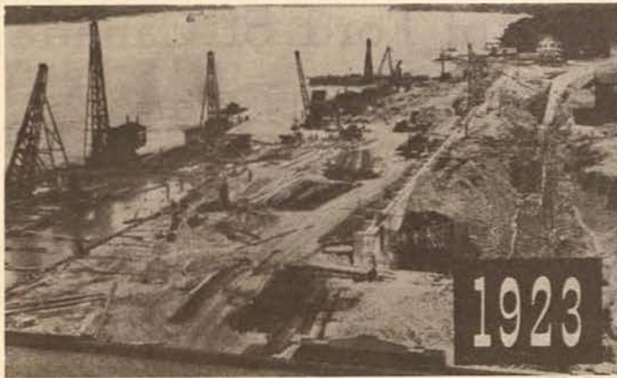
TYPICAL LANDMARKS at Ford-Windsor are the coal pile and the big Gantry crane. Preparations for their installation took place in 1923 when the fill-in was made for coal storage.
