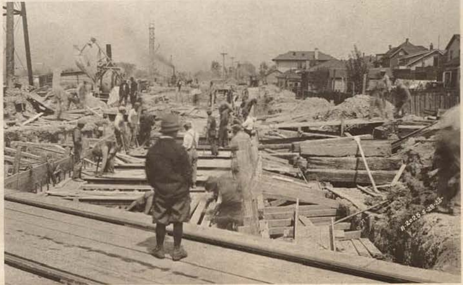
THE INTERESTED YOUTH watching Ford of Canada construction would now be middle-aged, as this photograph was taken in 1916 during erection of the sawtooth building of Plant 1.
