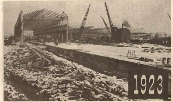
FRAMEWORK FOR PLANT 2 goes up in 1923. The picture, taken in March of that year, gives an idea of the tremendous cement foundations for the steel girder framework.
