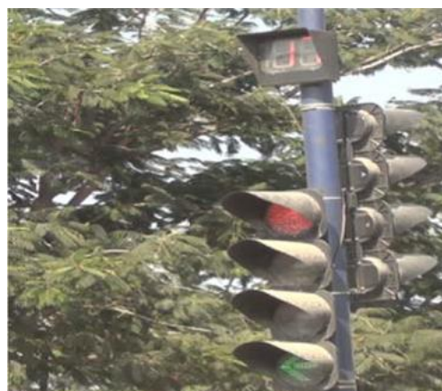
Figure 2-4. TSCT installed at traffic signals in India. (Source: Jatoth et al., 2020)
