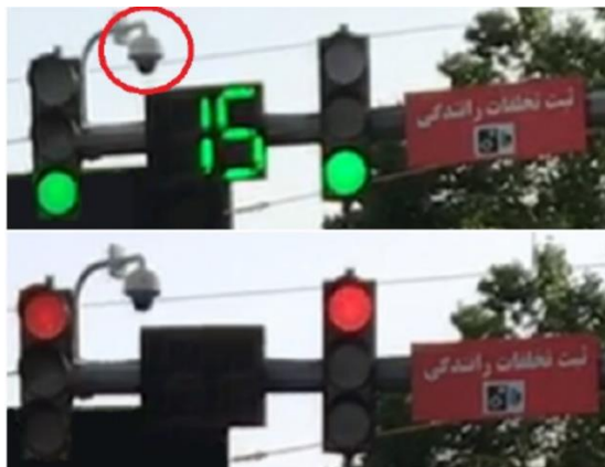
Figure 2-6. TSCT installed at traffic signals in Iran. (Source: Kashani et al., 2020)
