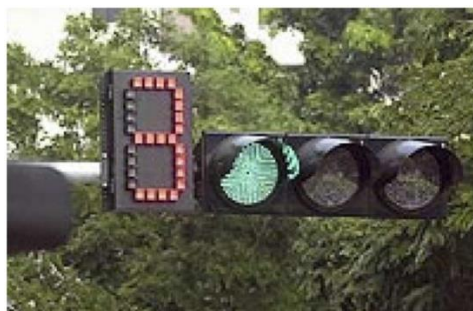
Figure 2-10. GSCT at traffic signals in Singapore. (Source: Lum and Halim, 2006)
