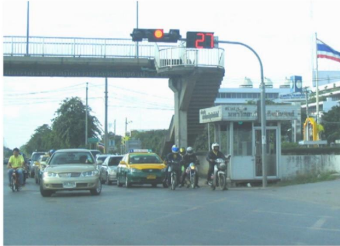
Figure 2-5. TSCT installed at traffic signals in Thailand. (Source: Limanond et al., 2010)
