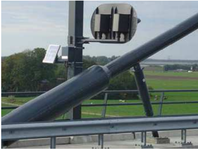
Figure 4-3 A viscous damper attached to a bridge stay cable
