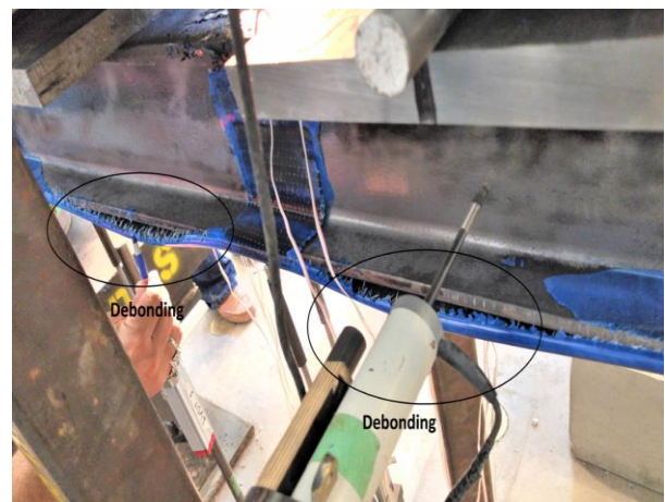
Figure 2.7: Debonding of BFRP fabric
