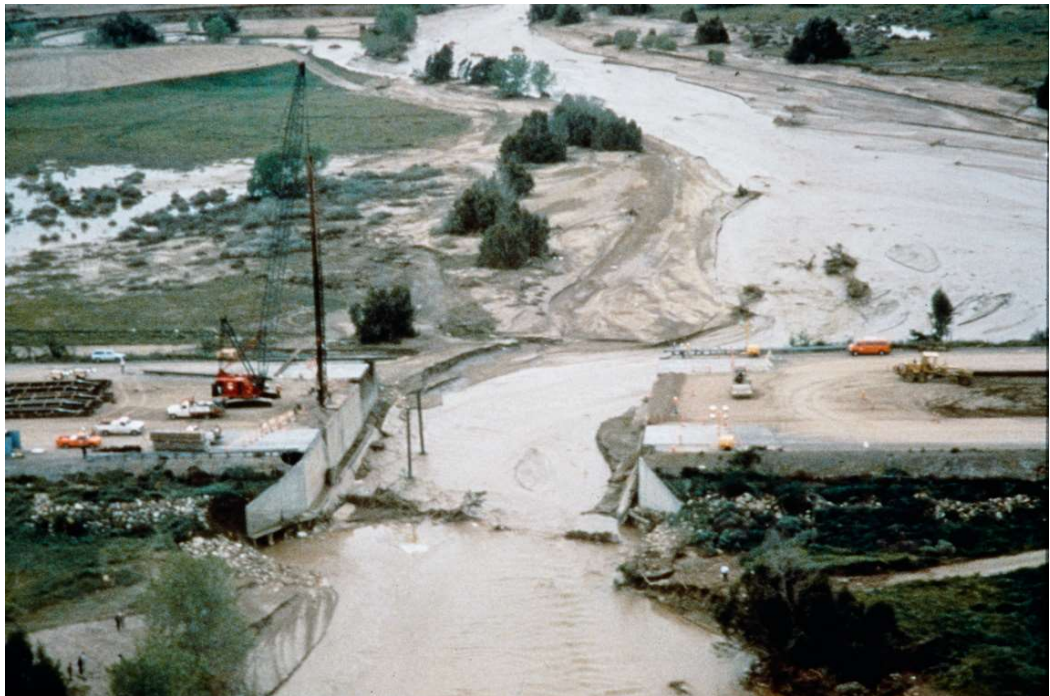
Figure 1.2: Arroyo Pasajero bridge collapse in CA, 1995 (Richardson 1995)
