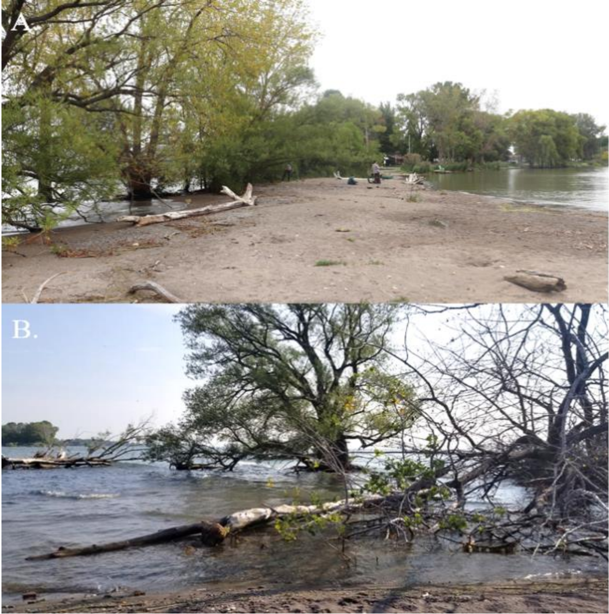
Figure 28: (A) Treeline at HB, before the rock revetment was installed, in September 2020. (B) Fallen trees and woody debris as a result of the retreating shoreline.
